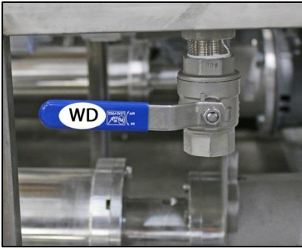
WD – Horizontal Left, valve is closed
